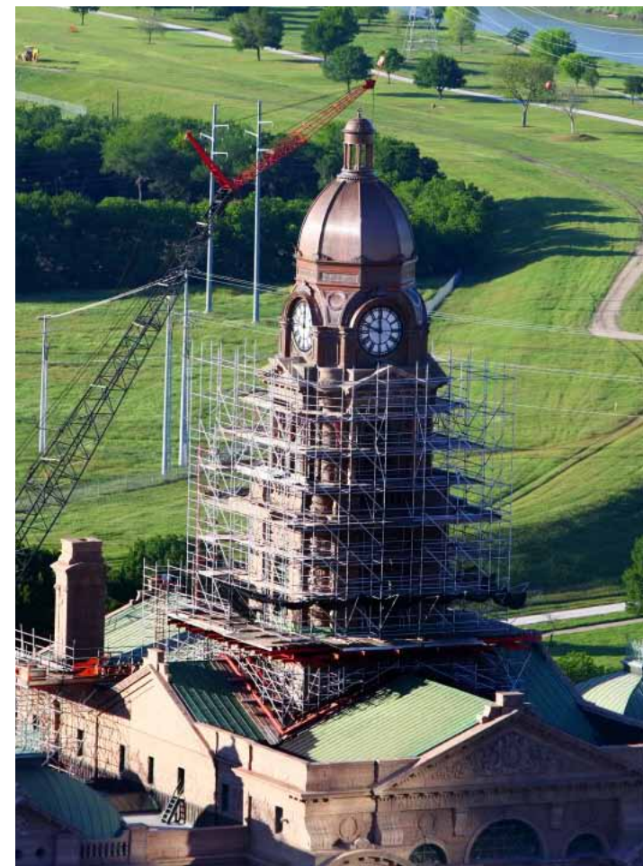
TARRANT COUNTY COURTHOUSE COPPER DOME WAS COMPLETELY REBUILT DURING RECENT RESTORATION EFFORTS
